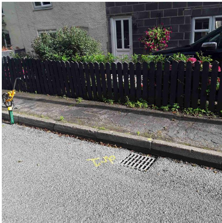
Photo from tablet device on site where flooding was reported on 17 August and a job was issued on 19 August to carry out jetting, investigation and any required civil works for repairs from gully to outfall to two gulleys. Note that water had subsided but officer determined there is still an issue.
